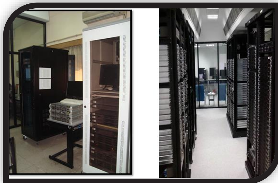
High performance computation facility at HRI
