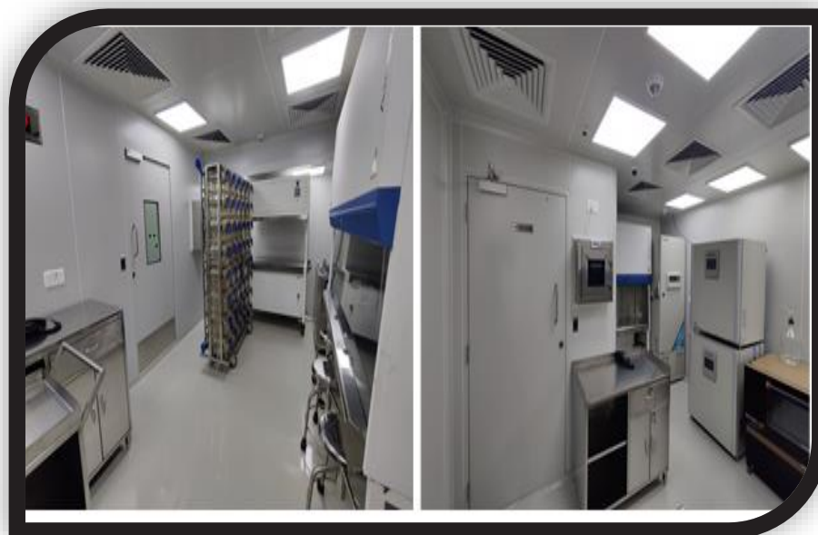
Biosafety Lab (Level III) at RMC-BARC
